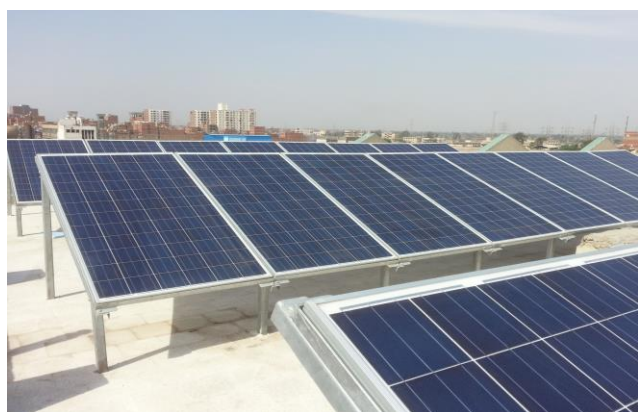
Fig. 5. View of the 18 kWp rooftop PV plant.
