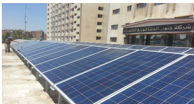
Fig. 4. View of the 18 kWp rooftop PV plant.
